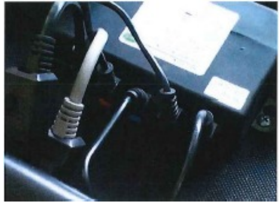
Lifting motor plug connected to control box.
